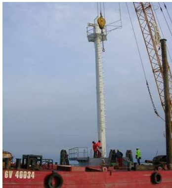
In addition, a radar tower for the STIM System was installed in Fusina.
